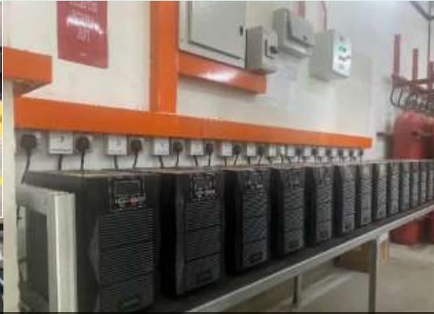
Back-up power installation for car park entry and exits
